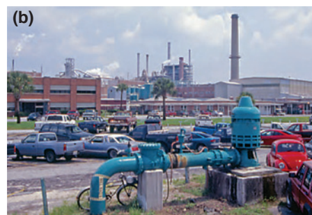
Large capacity well at a paper mill, St. Marys, Georgia. (Photo by Alan M. Cressler, USGS)
