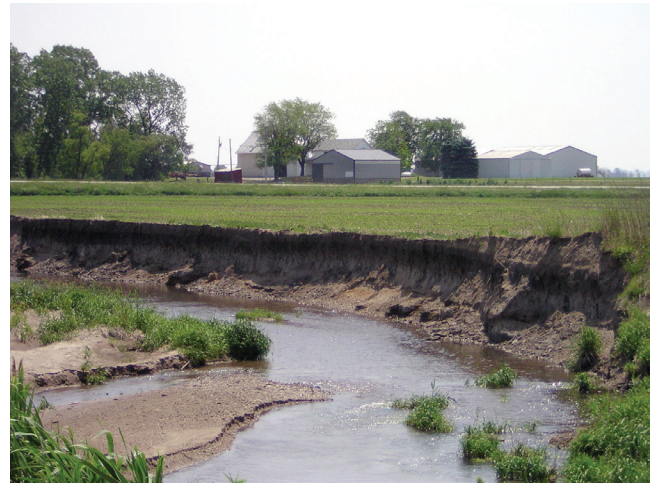
Figure 4.2. Lack of a riparian buffer and row cropping to the stream edge have led to stream bank failure and massive erosion along this stream in northwestern Indiana. Buffers of riparian vegetation stabilize stream banks and decrease sediment inputs to streams. (Photo courtesy of Todd Royer.)
