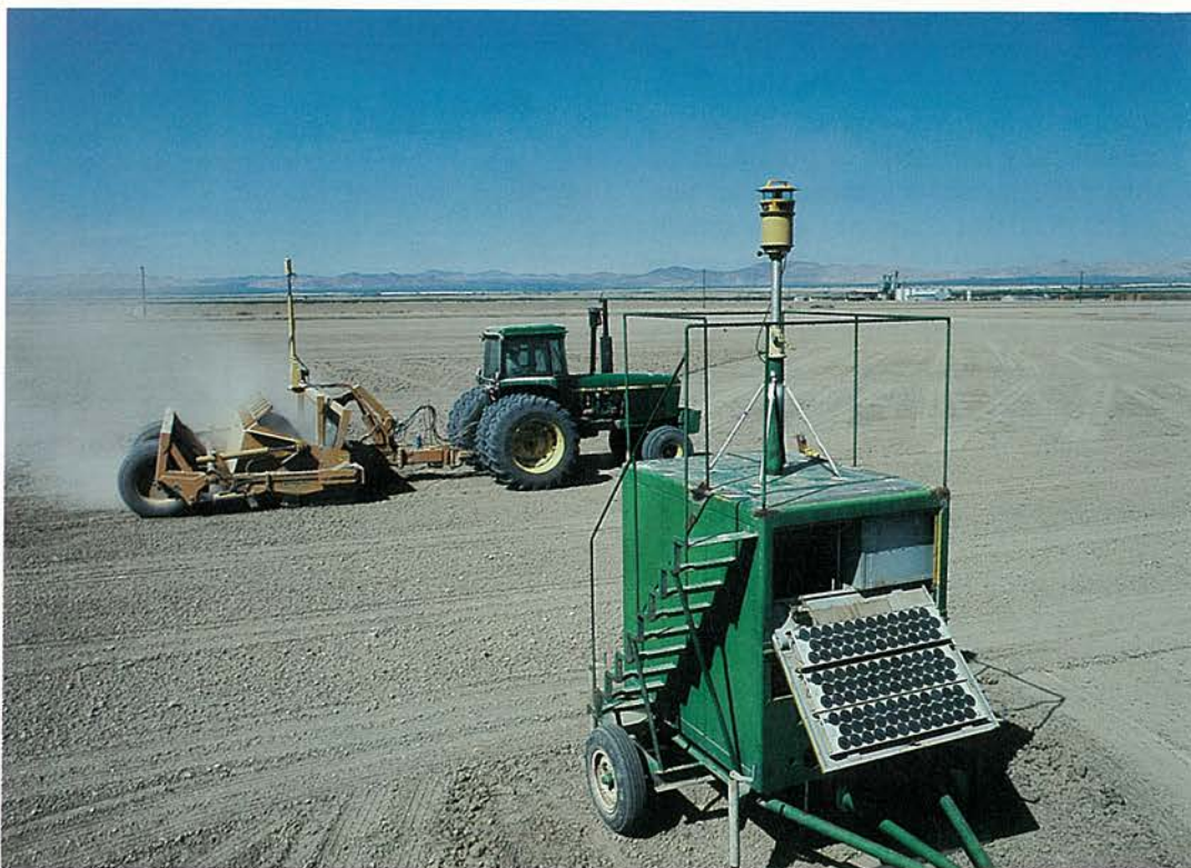
Figure 6.3. Laser-leveling of a level basin. Top photograph courtesy of Robert C. Bjork, Agricultural Research Service, U.S. Department of Agriculture, Beltsville, Maryland. Bottom photograph courtesy of A. R. Dedrick, U.S. Water Conservation Laboratory, Phoenix, Arizona.
