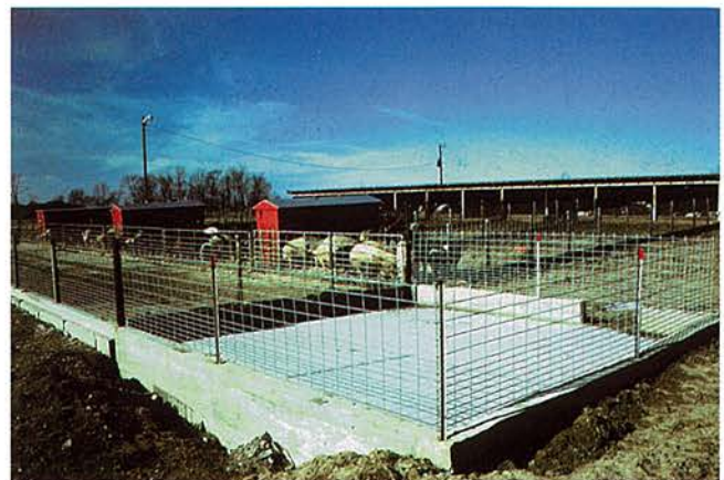
Figure 3.3. Concrete basin to settle solids during runoff from open swine lot. Photograph courtesy of Alan L. Sutton, Purdue University, West Lafayette, Indiana.
