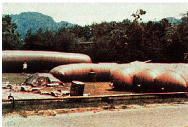
Figure 5.2. Biogas collection from anaerobic livestock methane digesters. Photograph courtesy of Don D. Jones, Purdue University, West Lafayette, Indiana.
