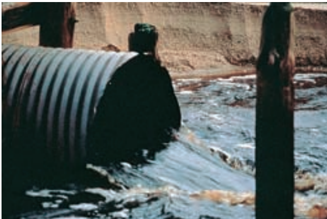
Figure 7.1. Storm water runoff flowing into Chesapeake Bay in the United States. Photograph courtesy of Chesapeake Bay Program, U.S. Environmental Protection Agency, Annapolis, Maryland.
